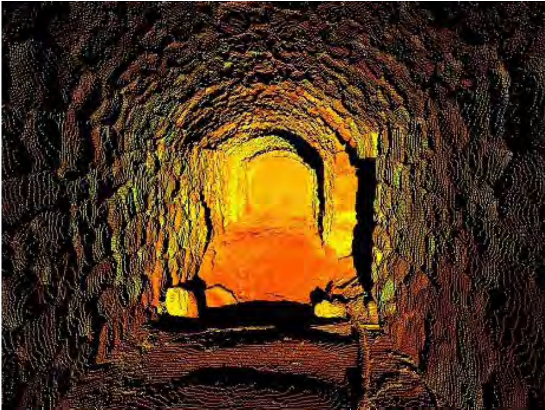
Fig. 5 a laser scan of the surviving accessible part of the drift tunnel
